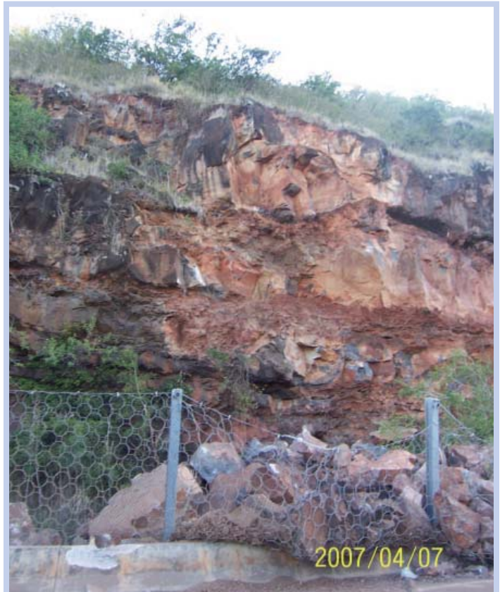
Condition after April 2007 rockslide showing crushed rockfall fence.
